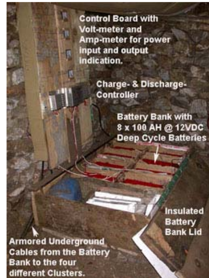
Figure 3-4: Battery Bank well insulated in a locally made wooden box, designed to last 8-10 years, including the load growth.
