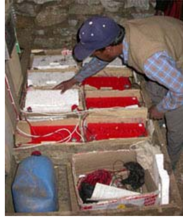
Figure 3-8: A project staff member teaches the local trainees how to check, clean and maintain the battery bank.
