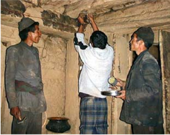
Figure 3-7: A project staff member trains the chosen local people in how to install and maintain the WLED lights, switches and house wires.
