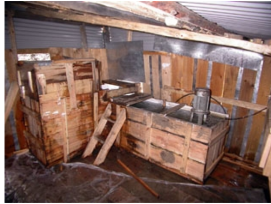
Figure 5: Inside the power house of the pico hydro power plant. The 1.1 kW generator is seen, with the wooden water canal, which cleans and streamlines the water for the propeller turbine's intake.
