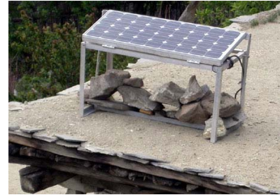
Figure 4-1: Cluster PV System
