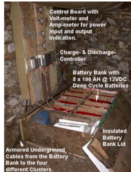
Figure 3-4: Battery Bank well insulated in a locally made wooden box, designed to last 8-10 years, including the load growth.
